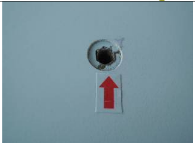
Pic.6 Screw installation is not smooth
